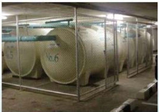
Hiclear installation at basement
