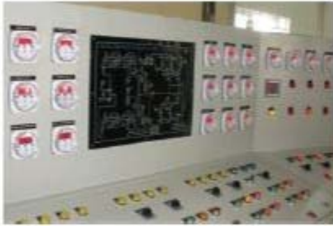
The Control Panel
