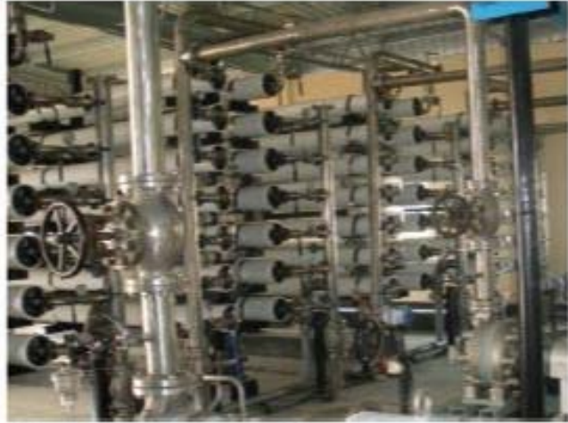
The Reverse Osmosis Plant
