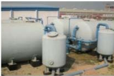
The Filtration units
